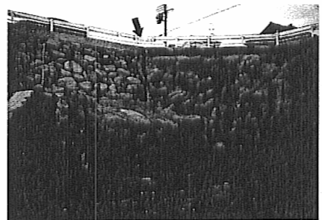
Photo 3 Damage Example at Facing Boundary of Rerforced Earth Structure
